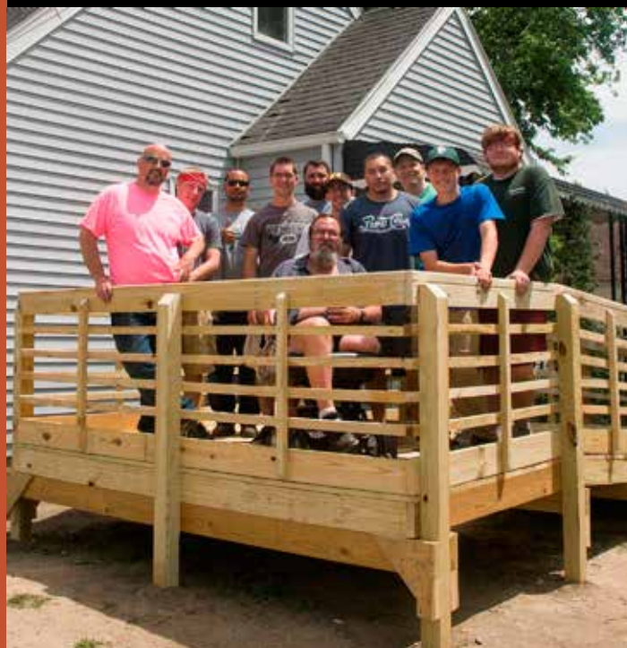
Herbie Myrice on his finished ramp with the Ability Center Ramp Crew and volunteers from the Catholic Heart Work Camp, one of our perennial ramp volunteer organizations.
